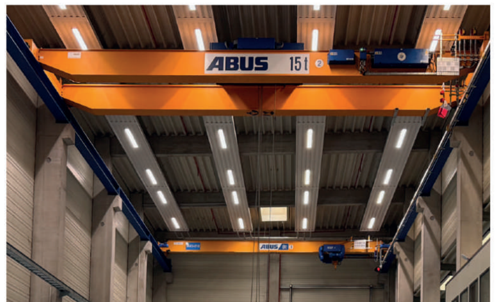
Crane systems: 8-tonne crane with a 38-tonne capacity
