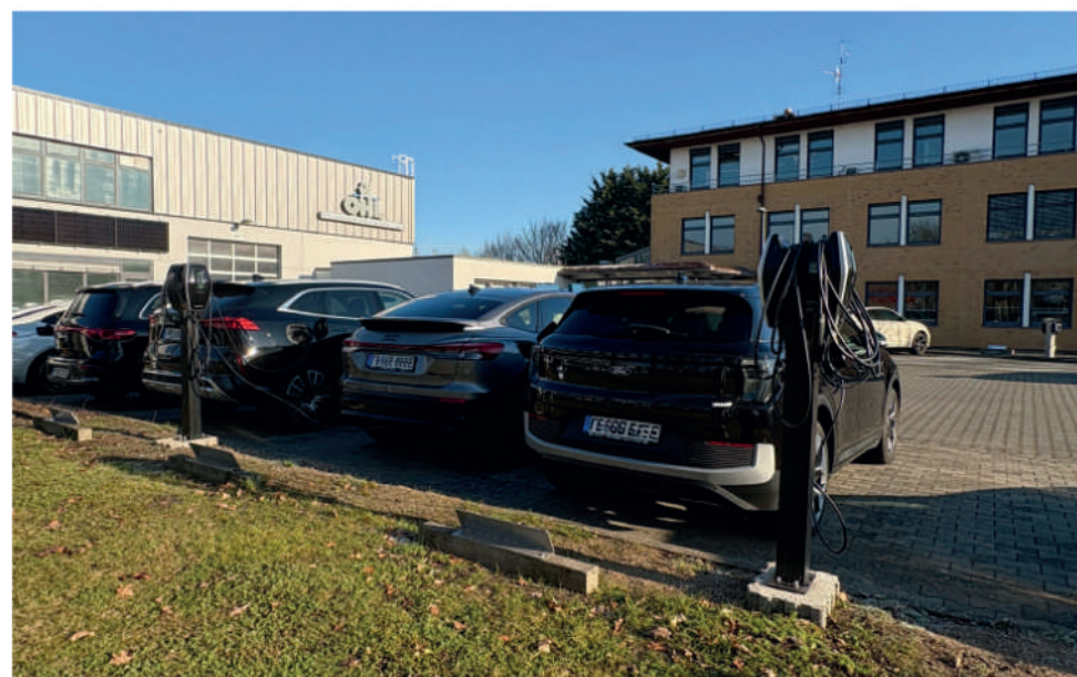
New EV charging points in the company car park
